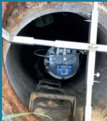
Wastewater sewer automatic sampler
